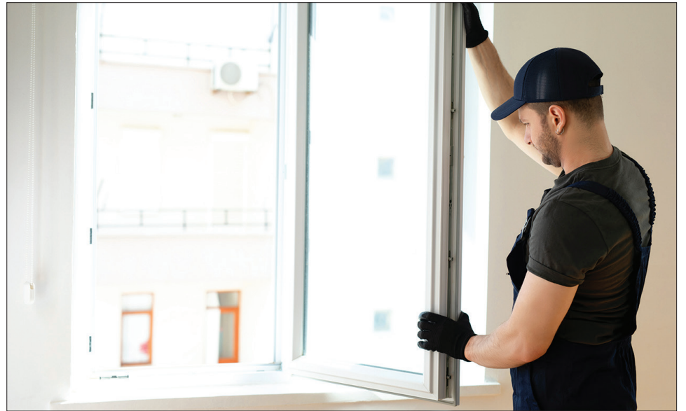
REPLACING WINDOWS is a job that requires advanced skill, and this is not a do-it-yourself project.
